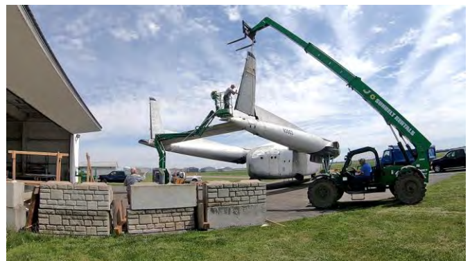
The assembly effort required the use of lifting equipment. Much of the equipment used by the team was provided by Sunbelt Rentals.
