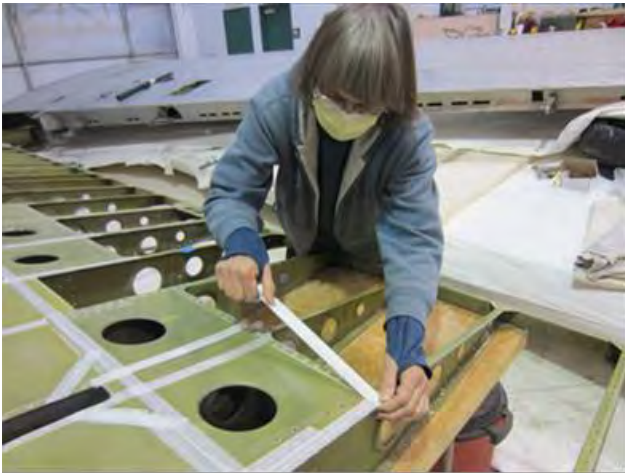
All of the fabric covered flight control surfaces (rudder, ailerons, trim tabs) had to be stripped, cleaned, and recovered. The rivets, and all sharp edges of the aluminum framework, were first covered with 1,900 feet of cloth tape.
